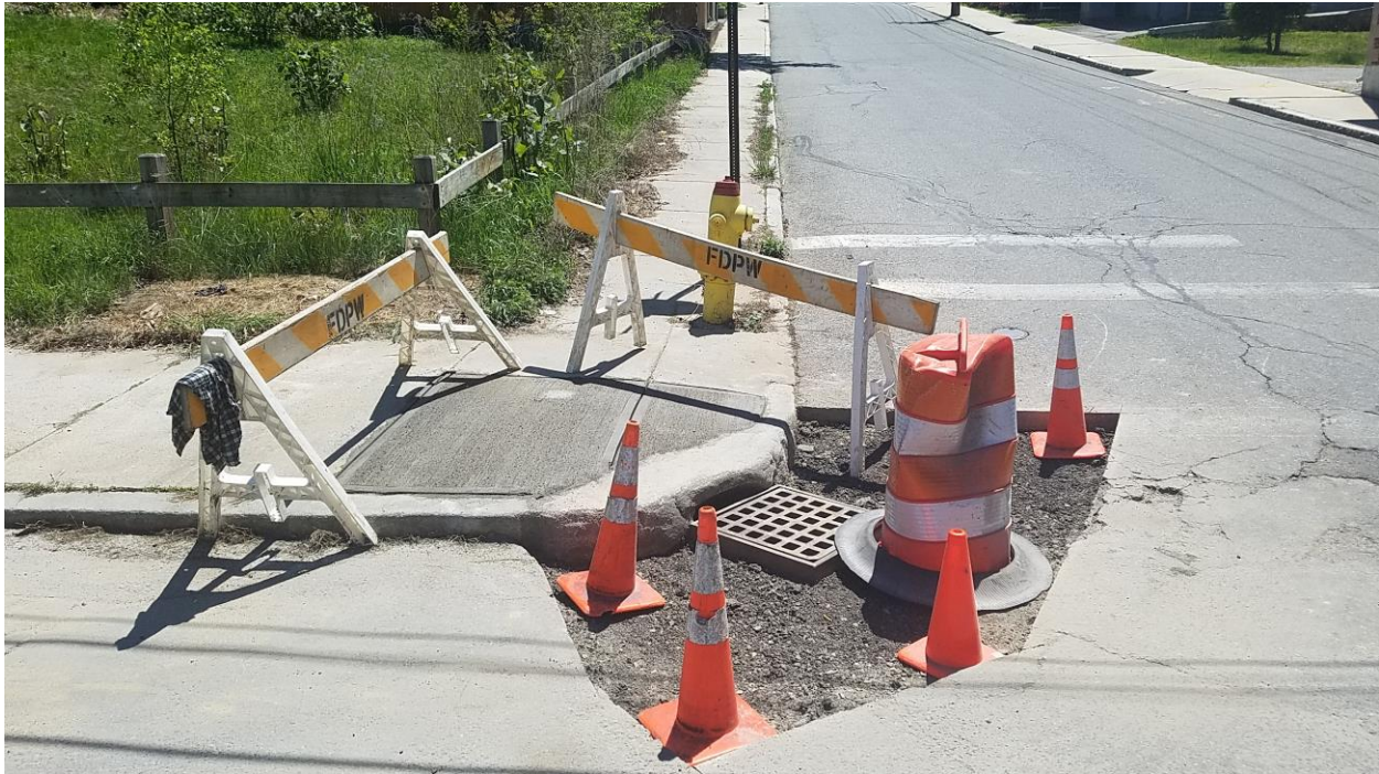
Figure 1 - CB rebuilt at Fairmount and Clarendon
