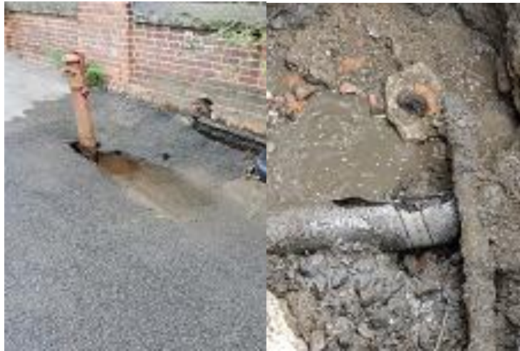
Figure 5 - Water main break - Daniels Street
