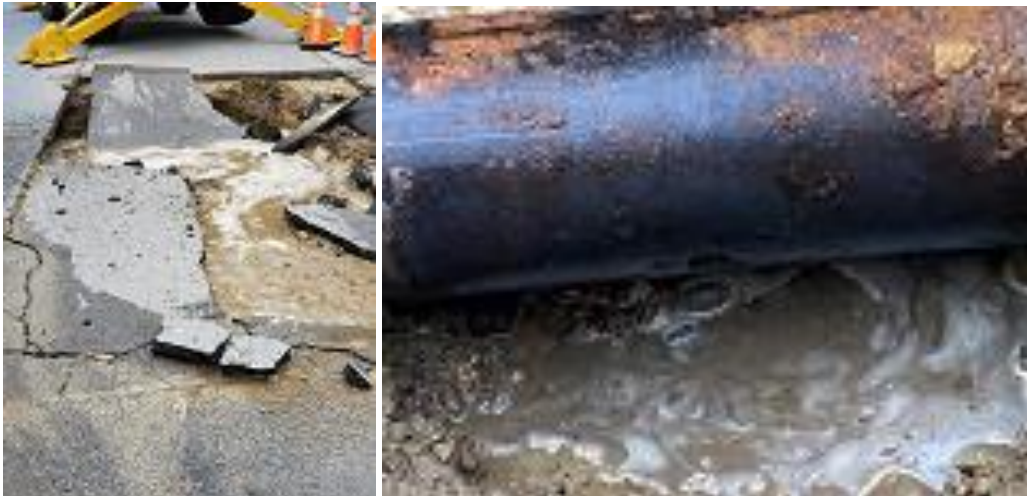
Figure 6 - Water main break - 21 Read St
