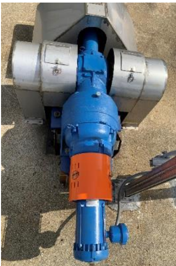
Figure 1: Primary Basin Speed Reducer.
