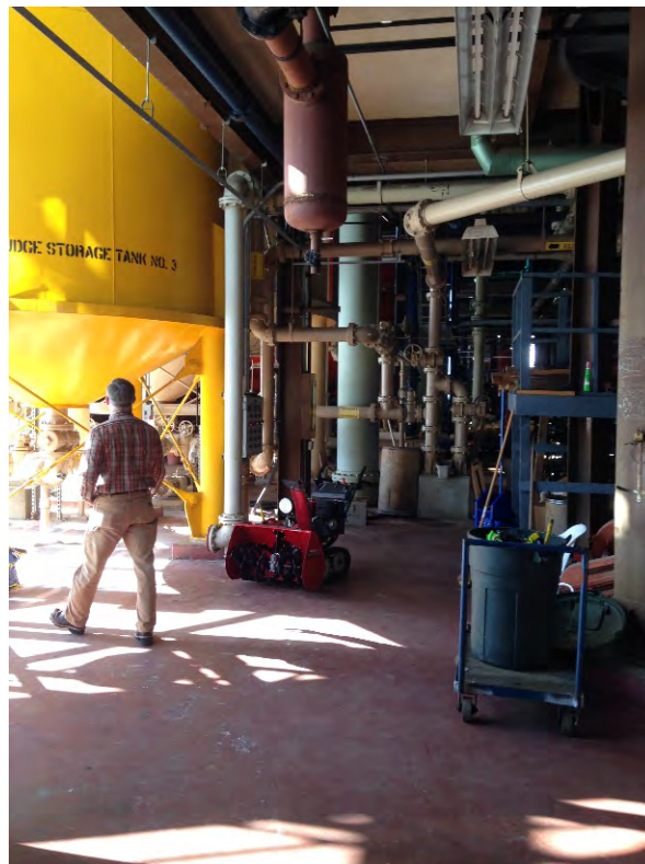
Photo 6: Steel sludge storage tank (typical 1 of 3) 3/6/2014
