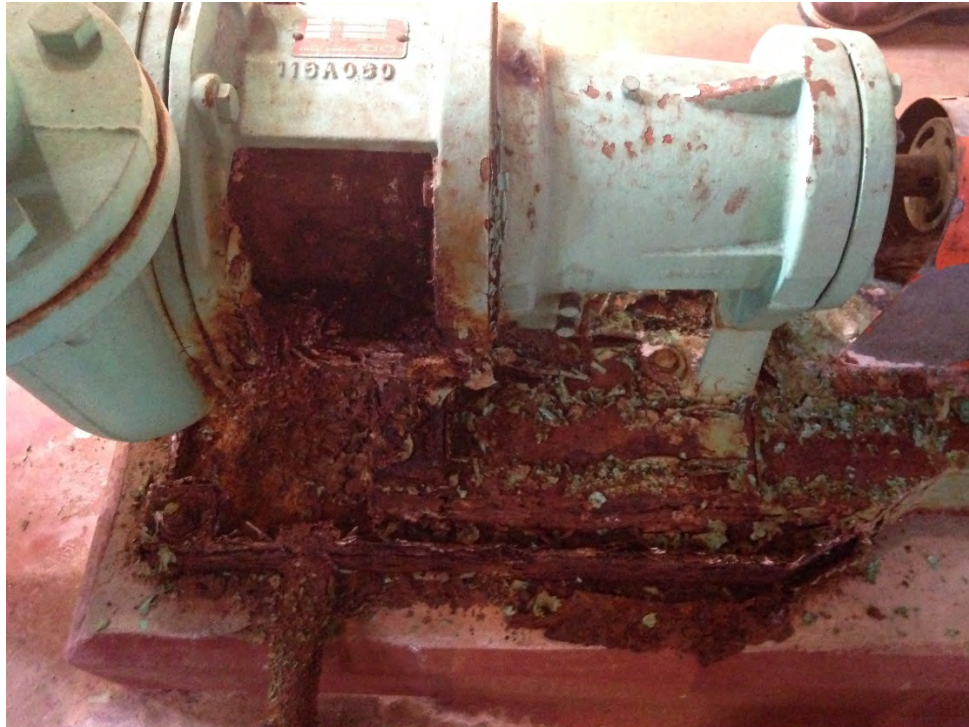
Photo 9: Filter pump, note corrosion and poor condition 3/6/2014
