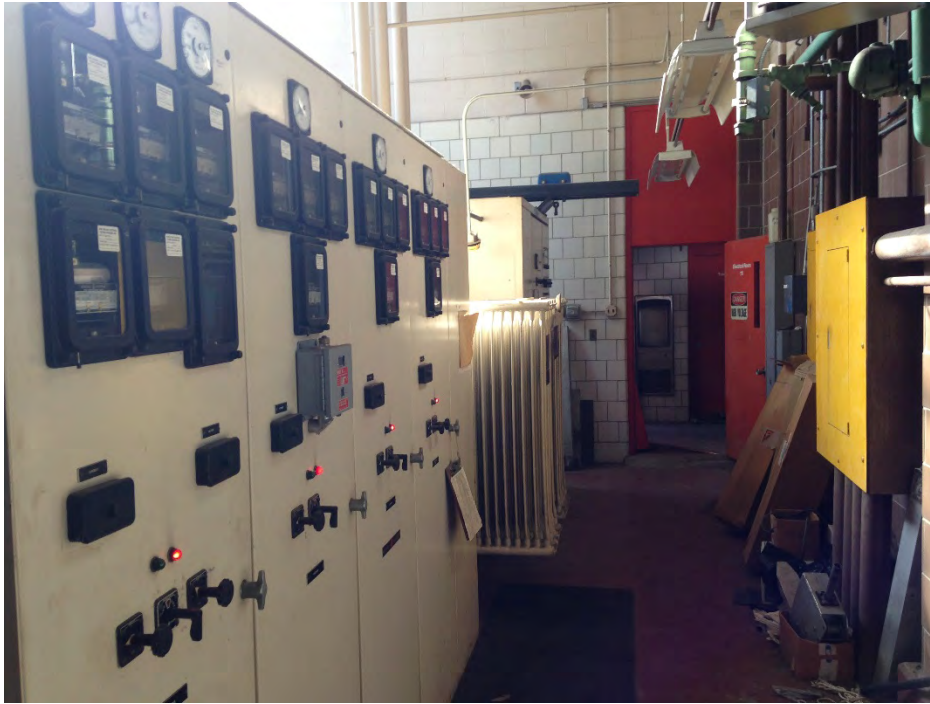
Photo 5: Main motor control center in electrical room of filter building 3/6/2014
