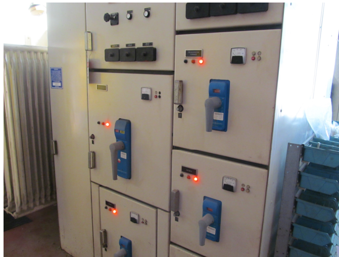
Photograph #3 – Indoor 480V, 2000A Switchboard
