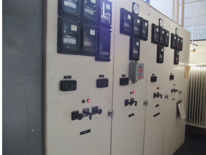
Photograph #2 – Indoor 4.16kV Switchgear and Transformer
