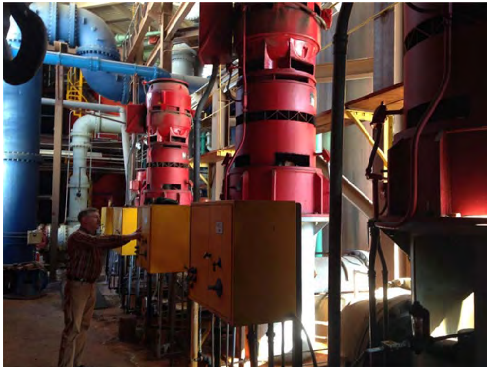
Photo 12: Vertical turbine pumps over wet wells on west end of filter building 3/6/2014
