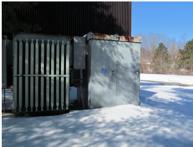
Photograph #1 – Outdoor 13.8kV Switchgear and Transformer
