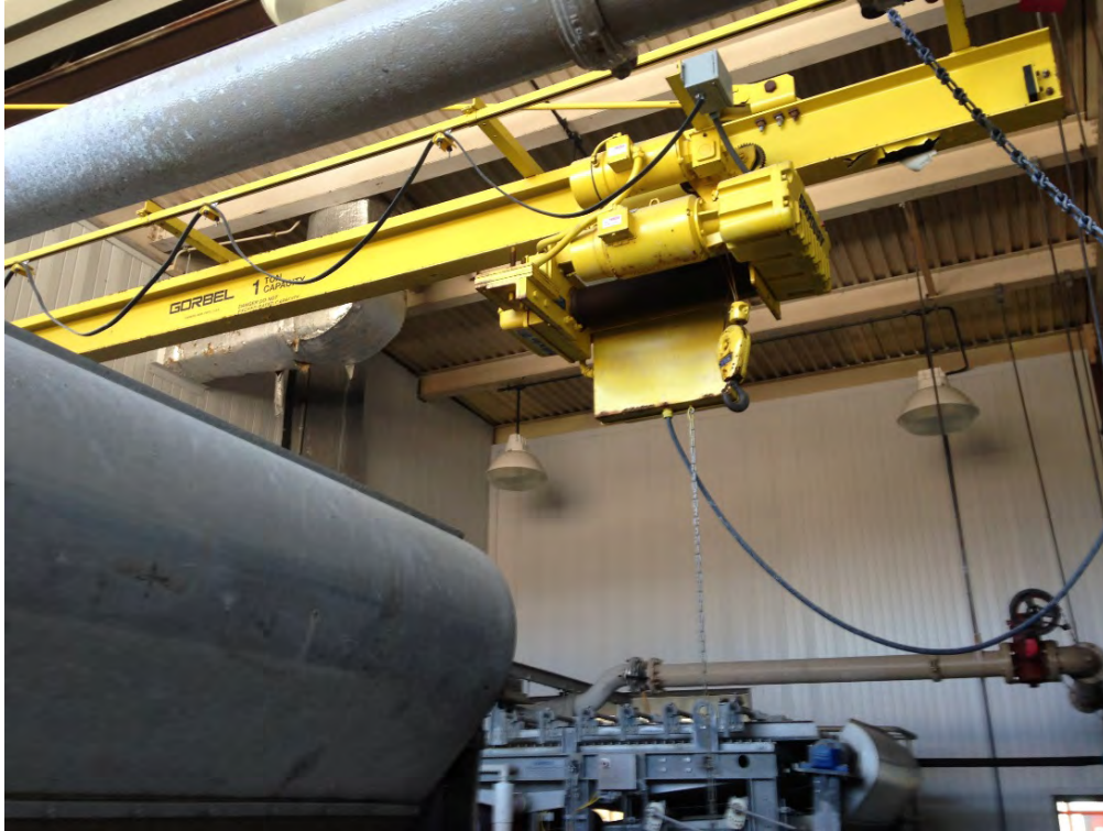
Photo 3: Gorbel® 1-ton overhead crane over belt filter presses 3/6/2014
